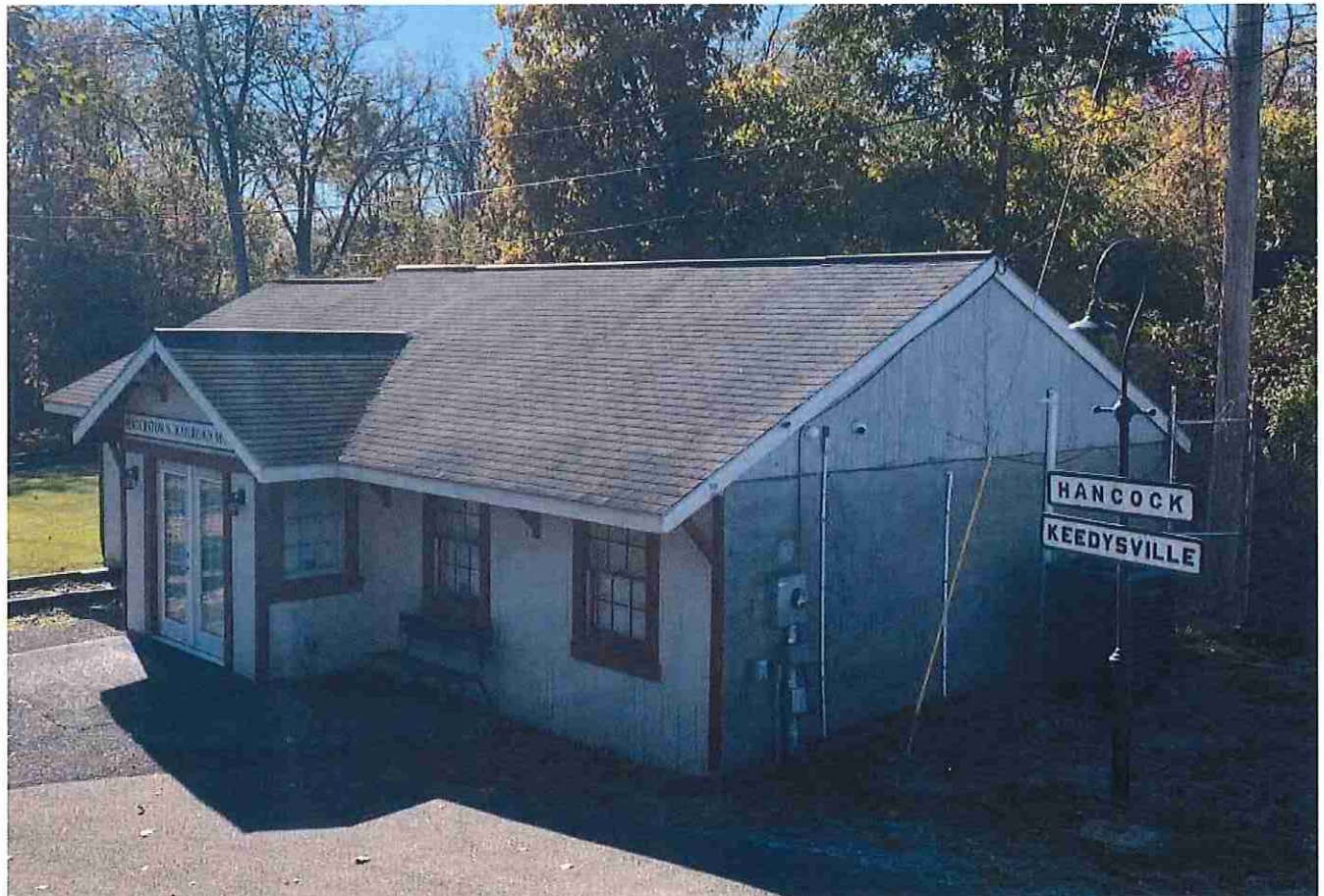
Asphalt shingles to be replaced with metal roof.
