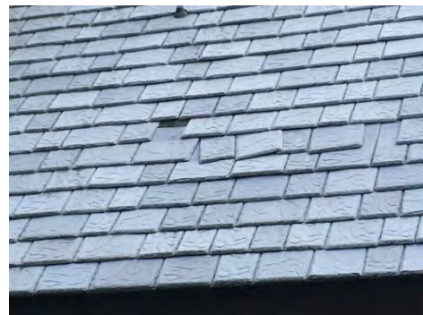
Repairing historic slate roofs can be very expensive, and craftsmen hard to find. (Staff Photo)
