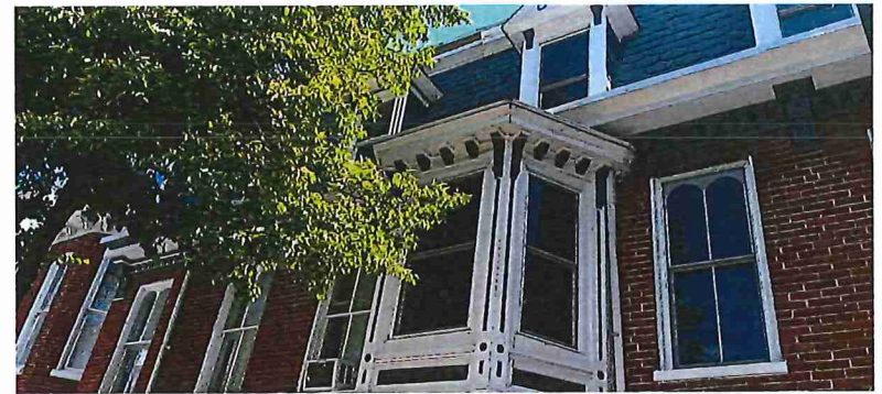
Slate material used on a mansard roof on the architectural front of a building. Is it real? Or is it rubber? (Staff Photo)
