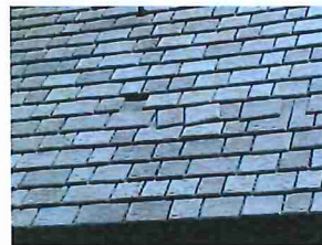
Repairing historic slate roofs can be very expensive, and craftsmen hard to find. (Staff Photo)
