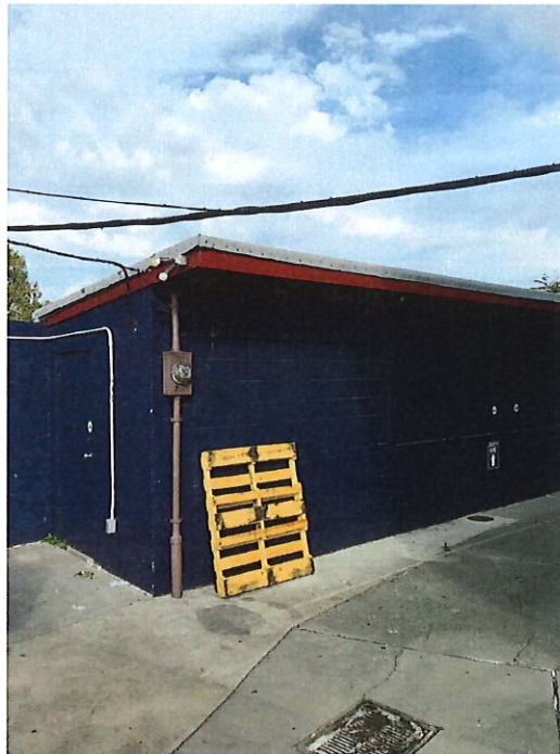
Concession building needs new roof
