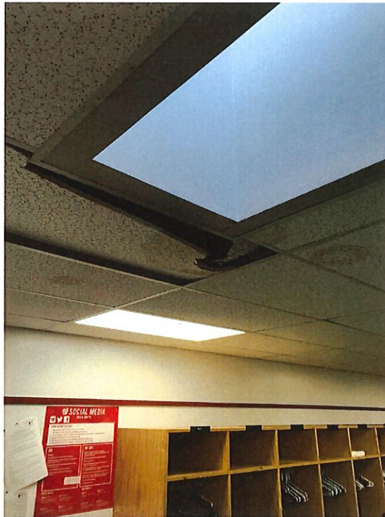
Damage from leaking roof in clubhouse
