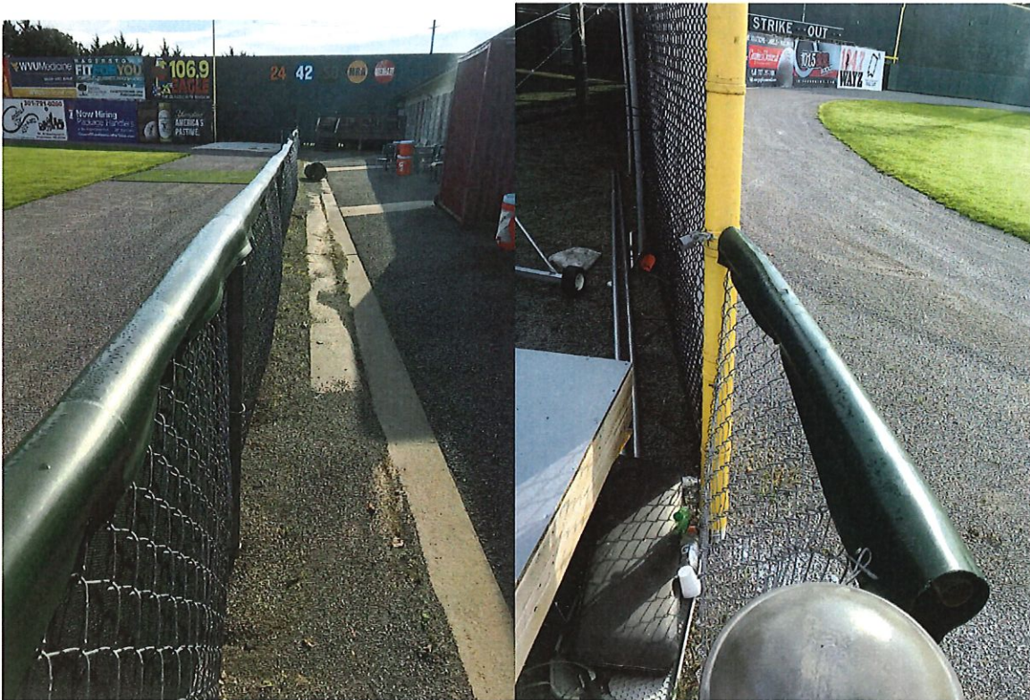
Replace field fence due to bows, breaks, and gates not operable
