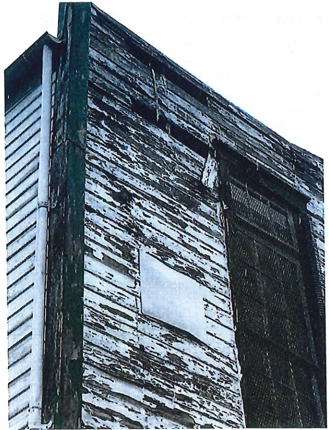
NE Corner water damage
