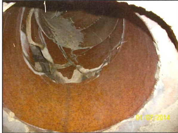
Figure 2 – Collapsing Pipe Discovered Using CCTV
